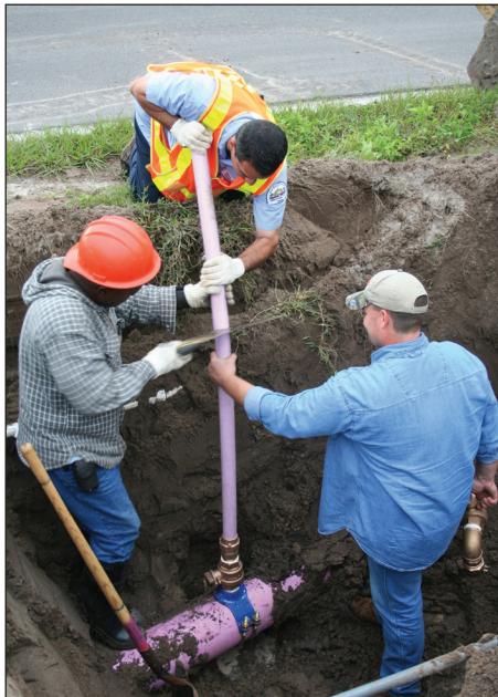
Purple pipes distinguish reclaimed water lines that serve 15,000 customers. The division has one of the largest residential reclaimed water systems in the country.
