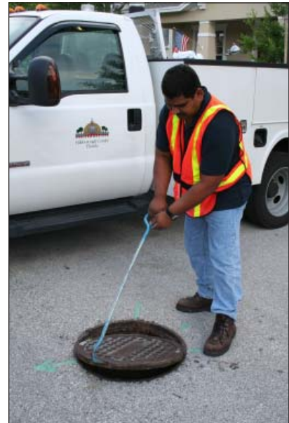
The utility counts more than 31,000 manhole covers in its system.
