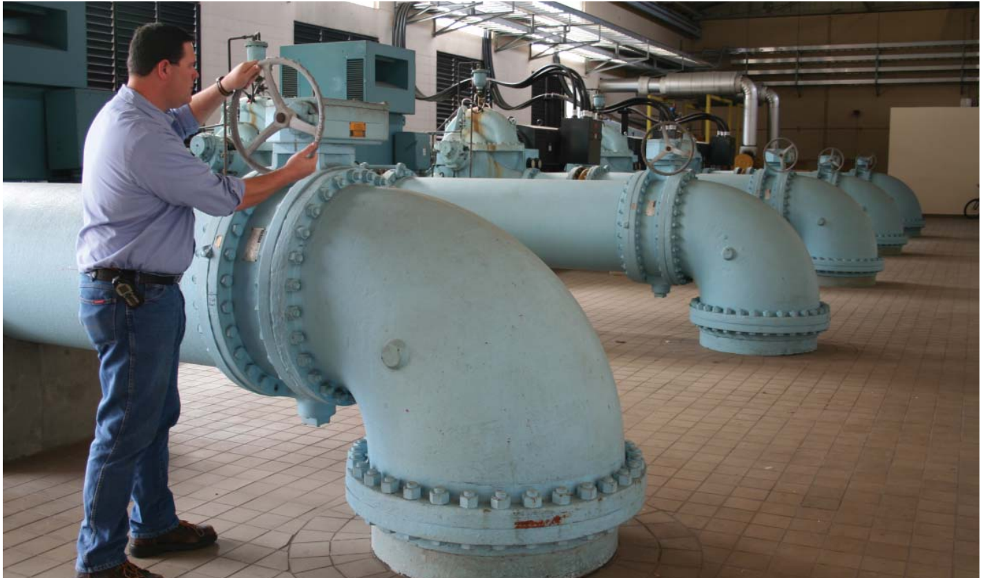
The pump room at the Lithia Water Treatment Facility. The plant supplies an average of 24 million gallons of high-quality drinking water a day to customers in central and south Hillsborough County.
